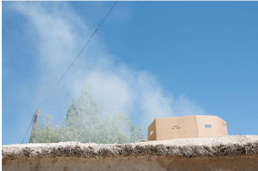
Figure 137: Prototype chimney in place over opening in roof succeeds in assisting the ventilation of the compartment.
